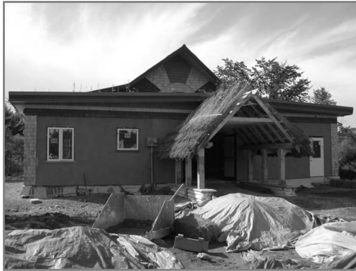
Camp Kawartha's new Environment Centre in Peterborough, Ontario, features prefabricated straw bale walls, earthen plaster, earthbag foundations, cotton batt insulation, a thatched roof over the entrance, rainwater collection and much more. Photo: David Elfstrom
